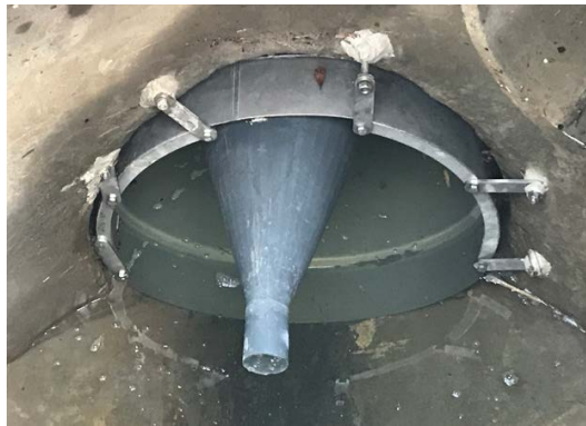
FIG. 11 DN600 - Custom designed valve inside manhole at Sulphur Beach, Northcote
