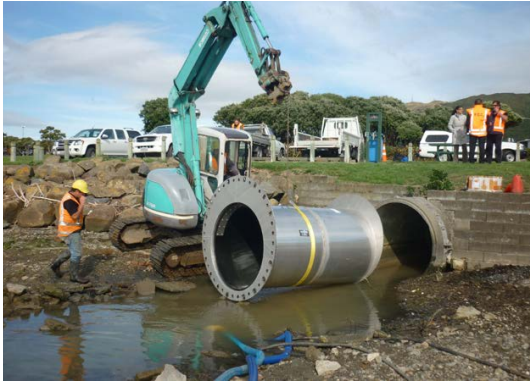
FIG. 10 DN900 Valve in DN1350 pipe, Porirua
