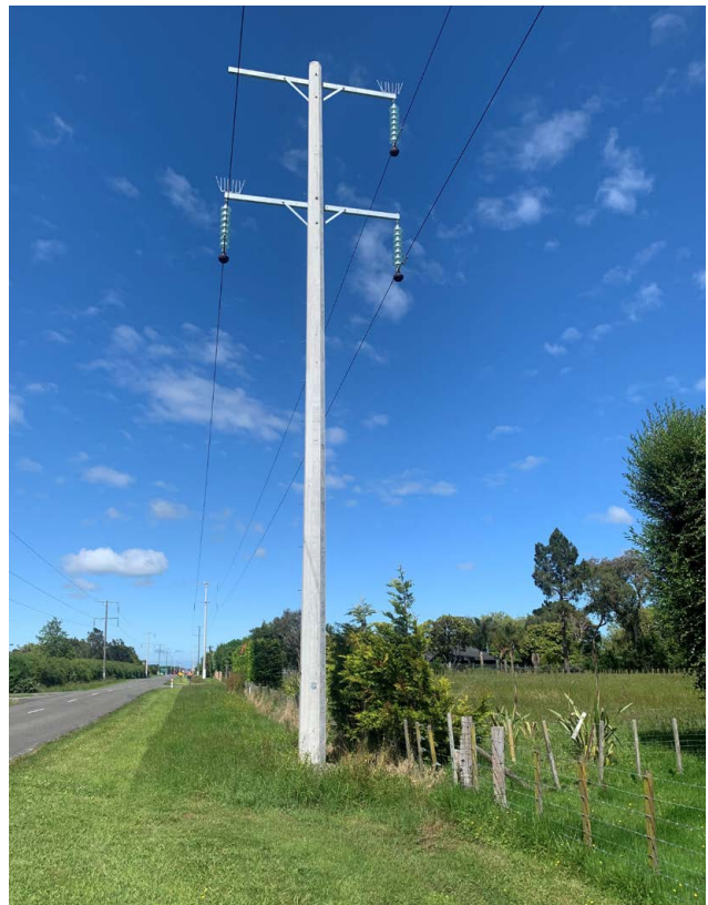
FIG. 3 | Octagonal power pole
