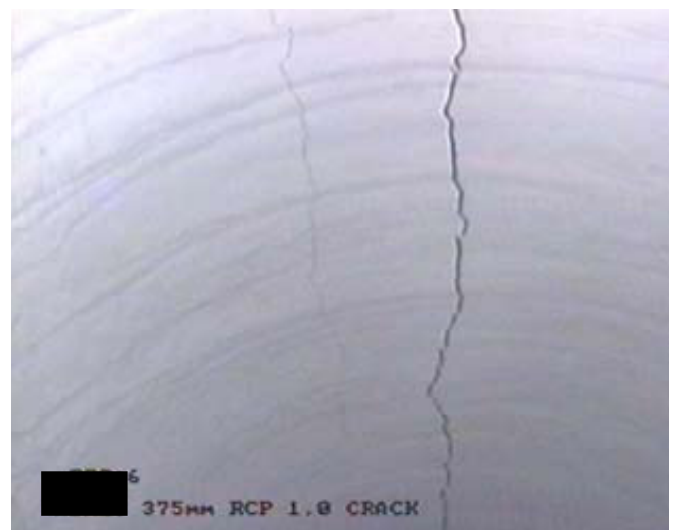
A 1mm crack at the obvert of a DN375 pipe, possibly caused by overloading of the pipe.
