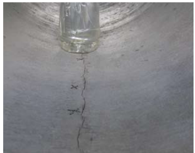
An 0.3mm crack at the invert of a DN450 pipe.
