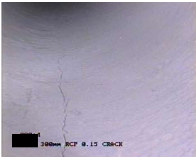
An 0.15mm crack at the obvert of a DN300 pipe tested for proof load. This is acceptable in accordance with AS/NZS4058
