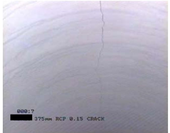
An 0.15mm crack at the obvert of a DN375 pipe tested for proof load. This is acceptable in accordance with AS/NZS4058
