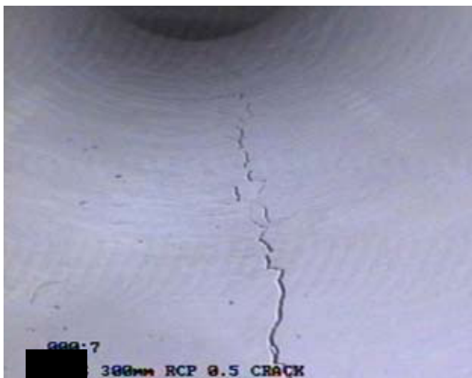
An 0.5mm crack at the invert of a DN300 pipe, possibly caused by overloading of the pipe
