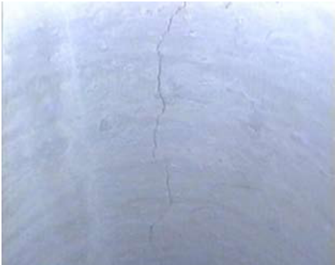
An 0.15mm crack at the invert of a DN300 pipe tested for proof load. This is acceptable in accordance with AS/NZS4058
